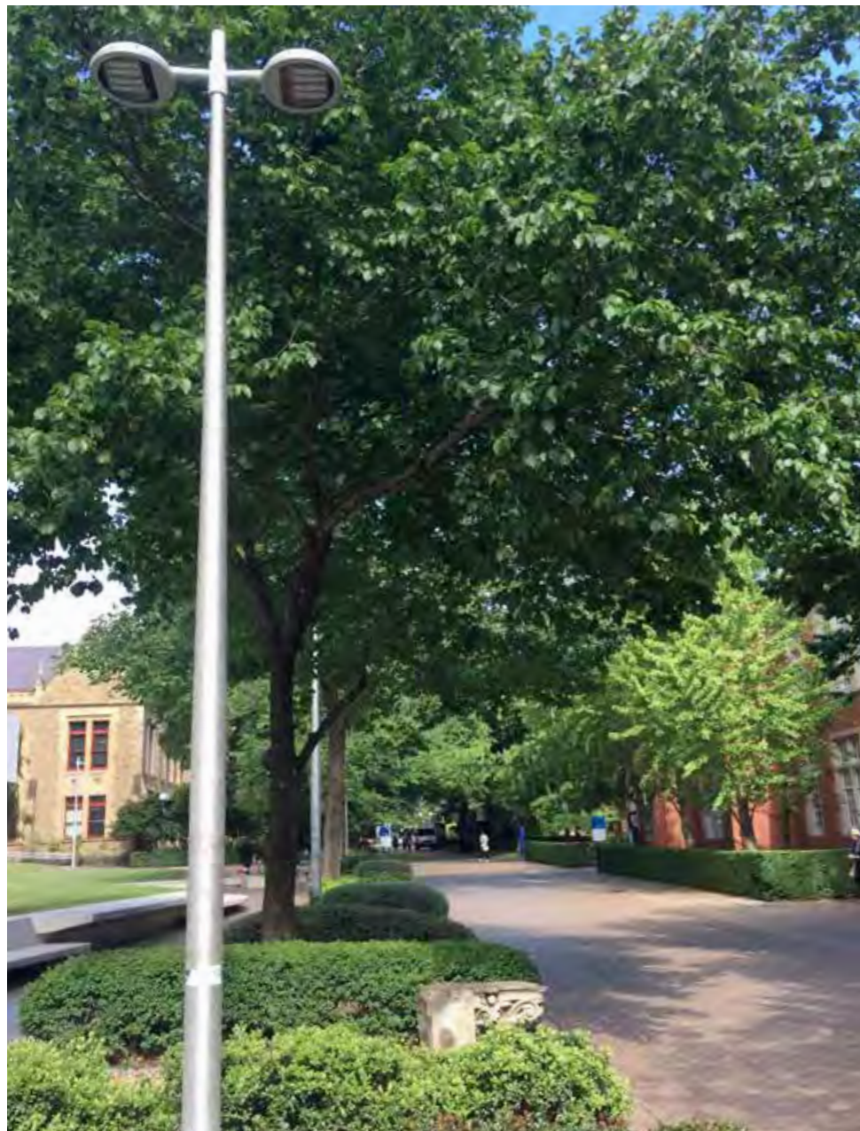
FUNCTIONAL LIGHTING: UOM STANDARD LED POLE LIGHT
