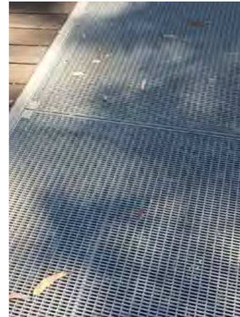
RAISED DECK: STEEL MESH WALKWAYS
